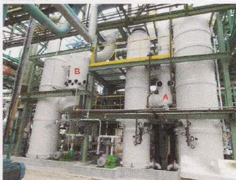
A – Venturi Scrubber System REITHER
